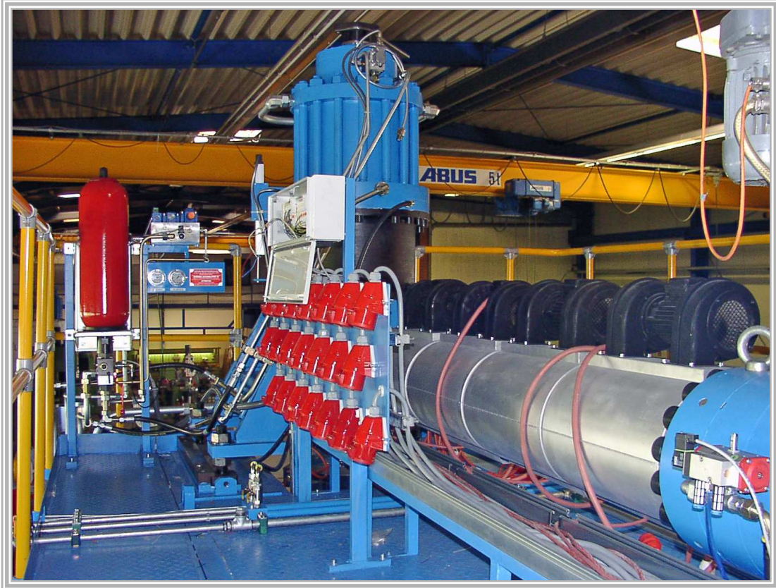
B-750: view of extruder platform
